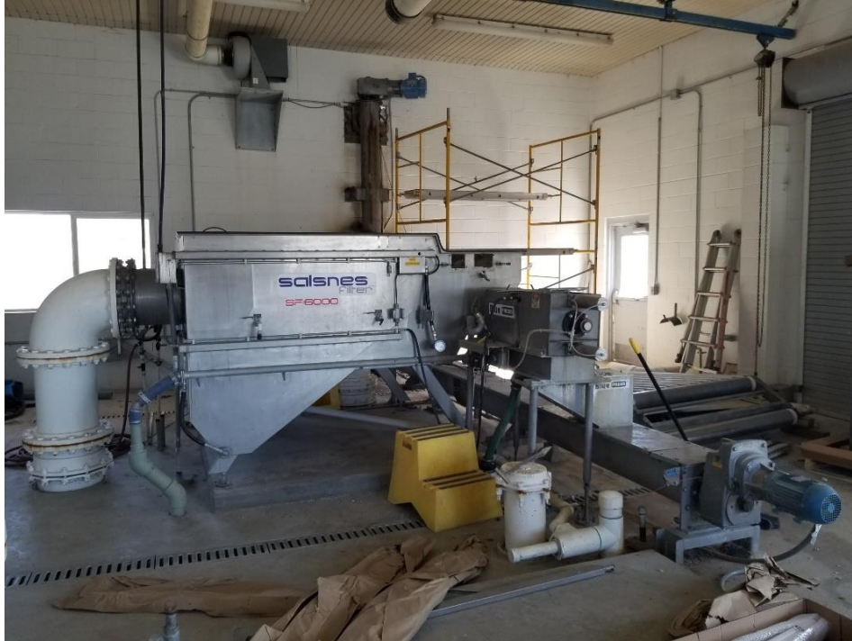
Figure 3-5: Salsnes Filter belt filter.
