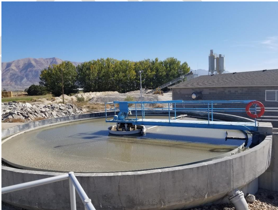
Figure 3-4: Primary clarifier w/ Salsnes Filter Building in the background.
