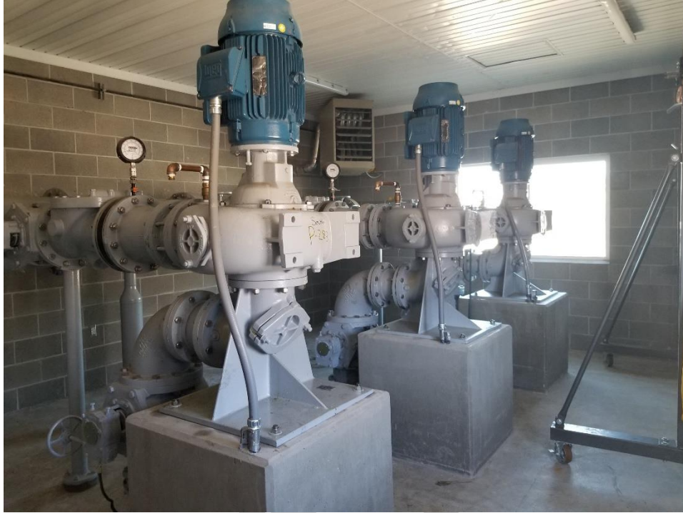
Figure 3-8: Internal recycle pump station.
