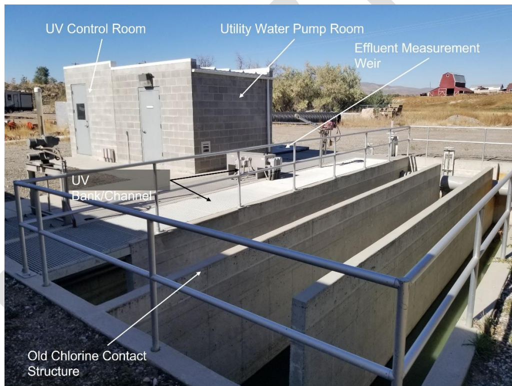
Figure 3-12: UV disinfection channel.
