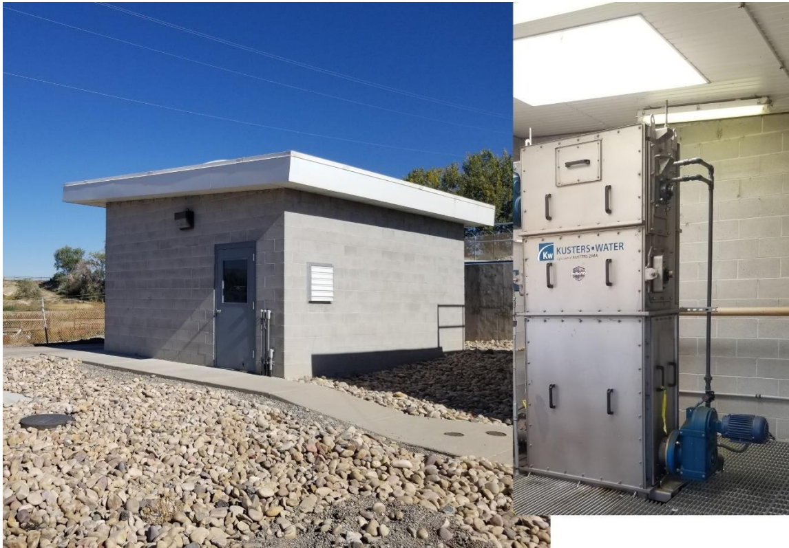
Figure 3-1: Headworks screening building (exterior) and screening equipment (interior).
