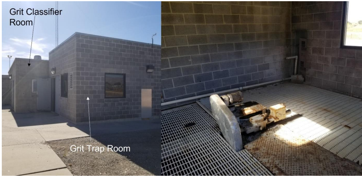
Figure 3-2: Headworks grit chamber building (exterior) and vortex mechanism (interior).
