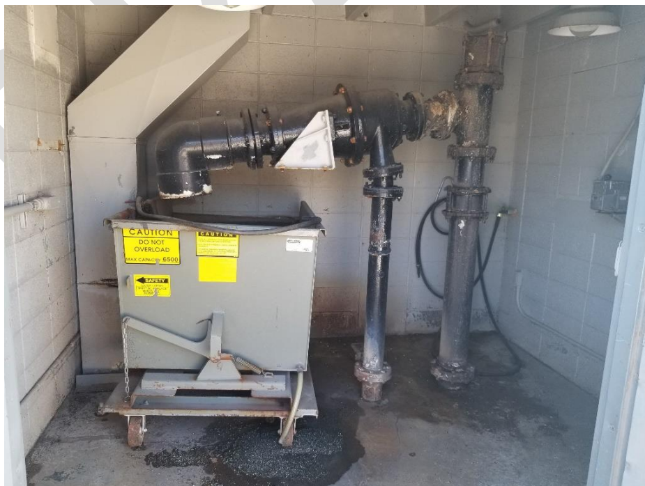
Figure 3-3: Grit classifier and dumpster.
