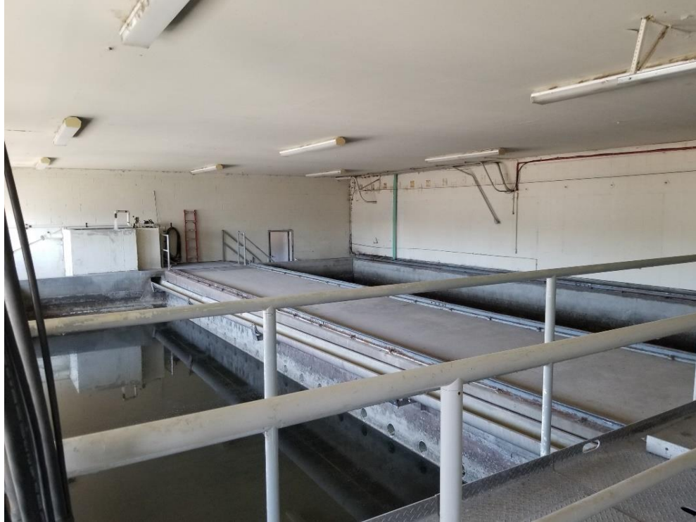
Figure 3-11: Sand filter basins.
