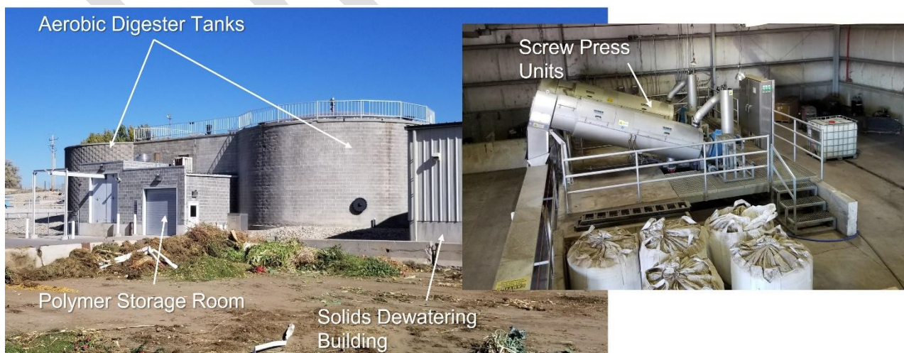
Figure 3-13: Aerobic digesters and sludge dewatering equipment.
