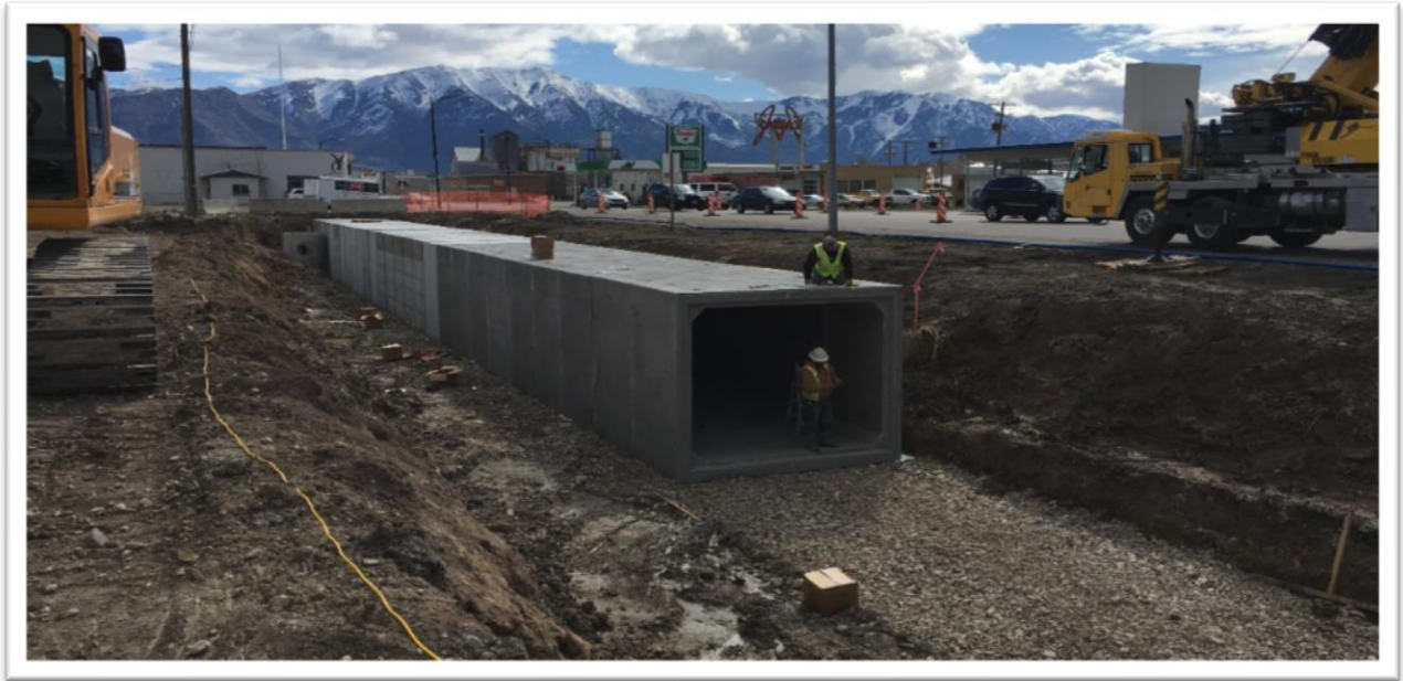
Photo of the canal being buried at the intersection of 400 West and Main Street (Tremont Center)
